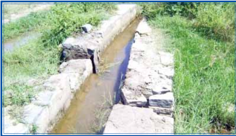
FIG: 19 DAMAGED GUIDE WALLS - TO BE RE-CONSTRUCTED/ REPAIRED
