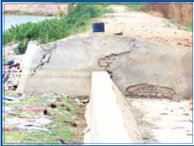
FIG: 12 DAMAGED ABUTMENT TO BE REPAIRED SIMULTANEOUSLY WITH BODY WALL
